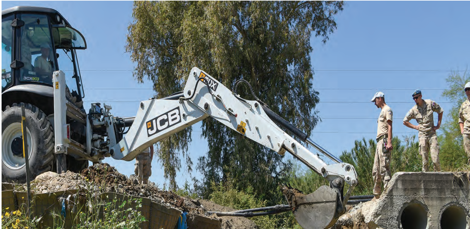
Mission Engineers construct, maintain and repair all facilities including camps, observation posts and patrol bases.
